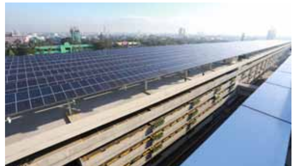
5,760 solar panels on the rooftop of SM North EDSA
